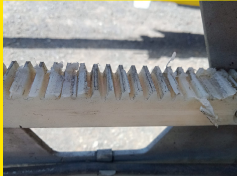
Worn nylon gear track on the H-beam.
