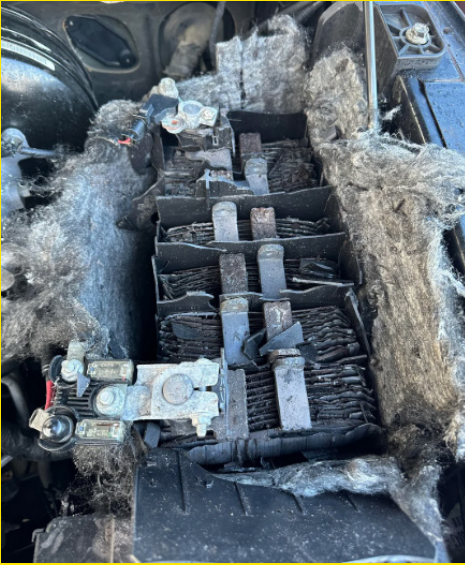
This battery exploded due to accidentally connecting the jump cables the wrong way around.
