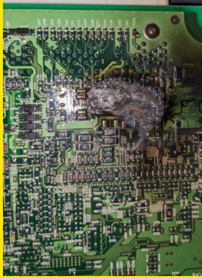
This is the circuit board of an ECU that was burnt out due to not following the correct jump start procedure.
